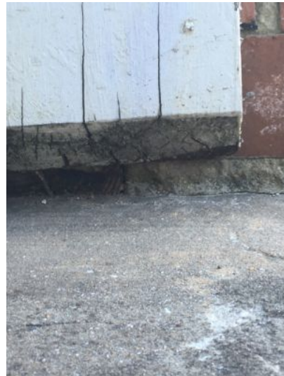
Bottom of garage door trim needs painting
