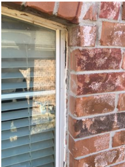
Caulk missing on back window
