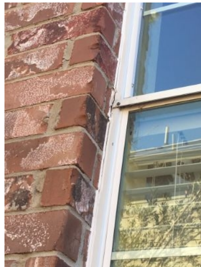
Caulk missing on front window
