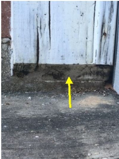
Bottom of garage door trim needs painting
