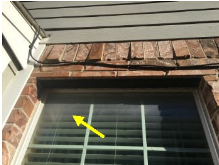
Upstairs window has lost thermal seal
